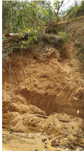
Fig 1.5 Seepage from toe of failed slope
