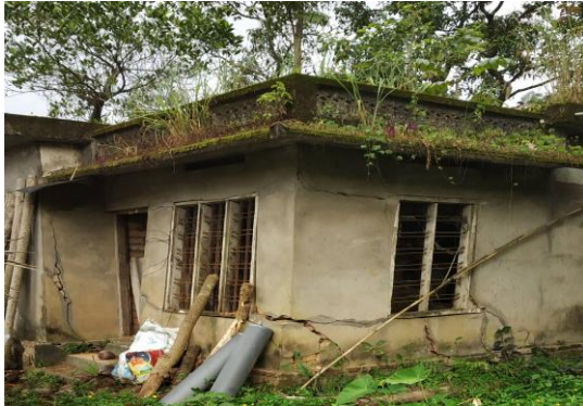
Fig 1.2 Houses which developed structural cracks at Santhigiri
